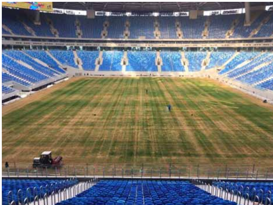
Initial pitch failure in 2016 and 2017
